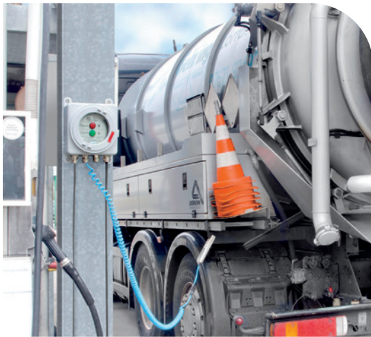
Active grounding for tanker trucks
