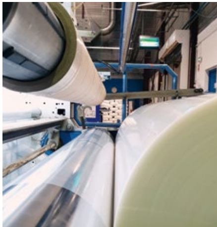
Installed flexION air discharging bar on the winder
